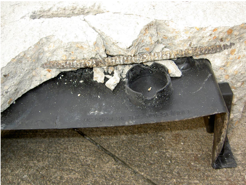
Figure B-8. Close view of rebar.
